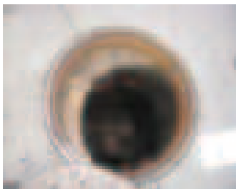
Figure 2.39 Offset of manhole block
